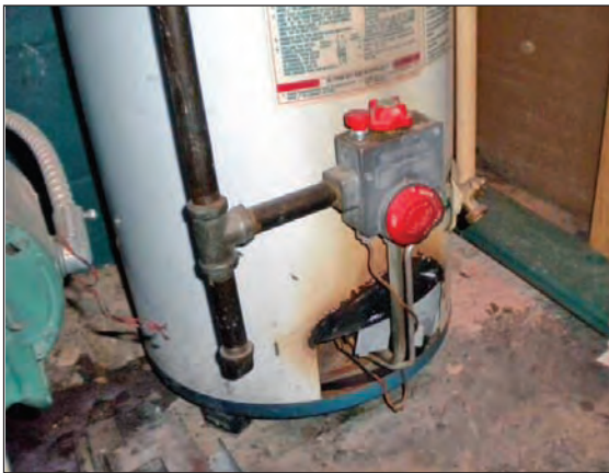
Evidence of flame roll-out.
